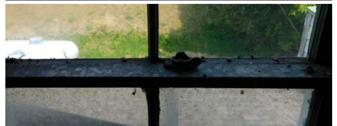
Figures 18-19 Details of north elevation second-story window. Note surface cracking at stile and rail joints, sill, and meeting rail.
