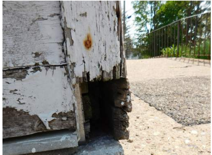
Figure 13 Deteriorated southwest corner boards.
