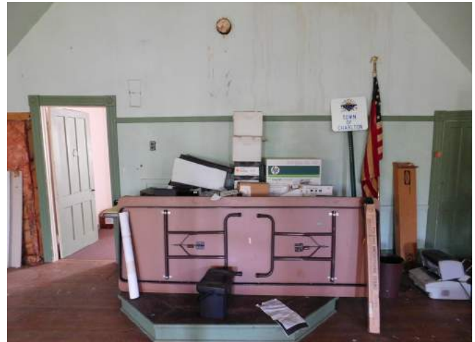
Figure 29 South wall of second floor hall. Note the chair and head rails and the water staining on the upper portion.
