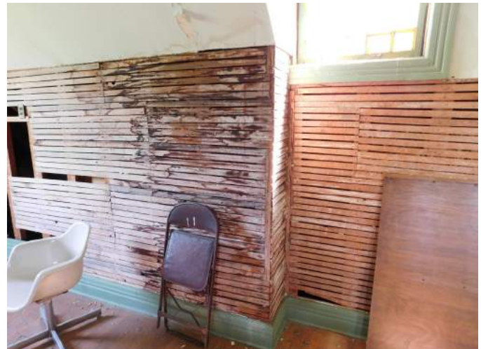
Figure 30 East wall of second floor hall. Note the water-stained lath and the historic baseboard.
