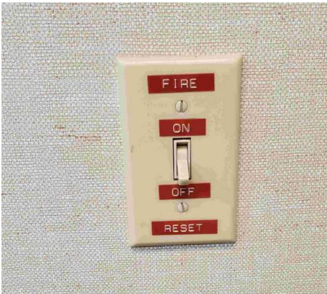
Figure 55 Fire Alarm Switch
