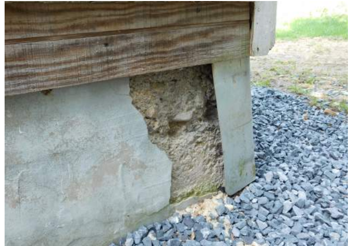
Figure 6 Spalling on rear addition concrete foundation.
