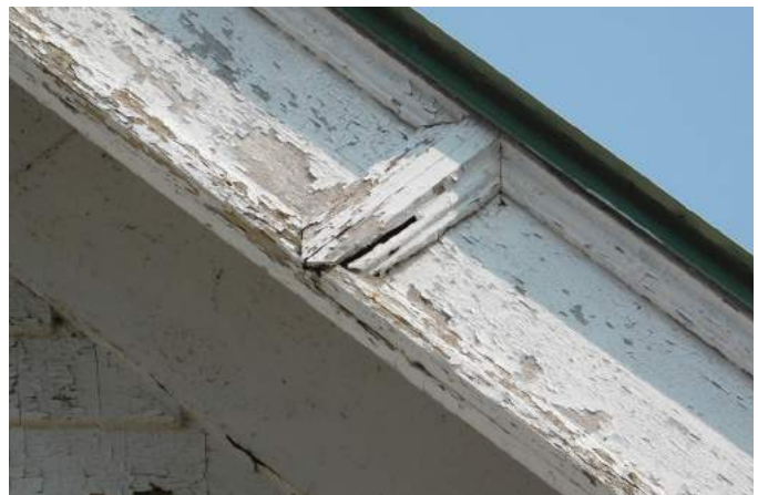
Figure 14 Rotted fascia trim element.
