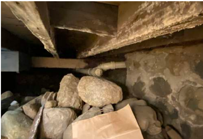
Figure 4 West foundation wall and decaying floor framing.
