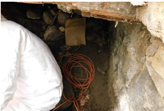
Figure 5 North foundation wall and rotted floor framing.
