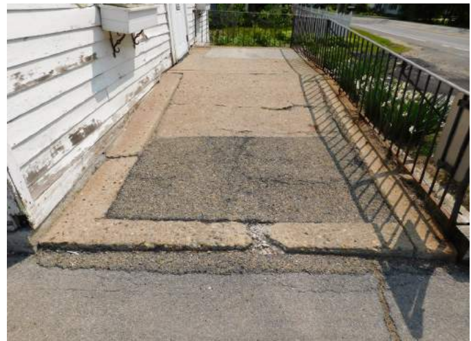
Figure 22 Cracked and disintegrating concrete ramp with asphalt patch. Erosion of binder and loss of aggregate as well as contact with corroded metals has weakened the structure and caused cracking and deterioration.
