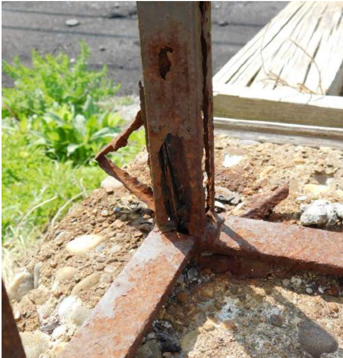
Figure 23 This heavily corroded iron railing post has damaged the concrete at its connection.
