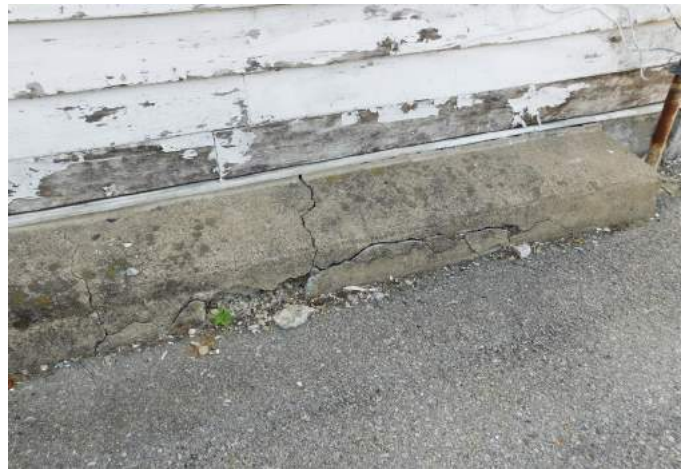
Figure 7 Cracked concrete wash along west foundation wall.
