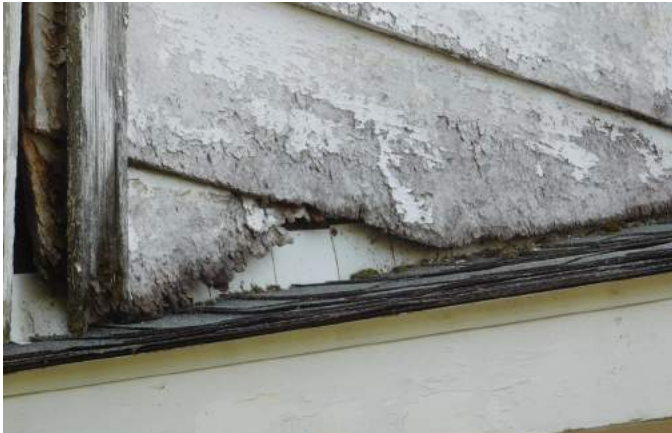
Figure 11 Deteriorated rear addition parapet wall cladding.
