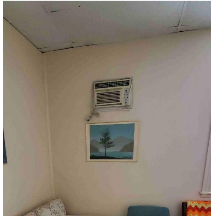
Figure 41 AC Unit in Lounge
