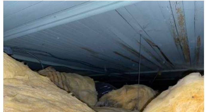
Figure 33 Concealed historic wood board ceiling above drop ceiling in main hall of first floor. Note the perpendicular trim pieces forming panels and the paint loss and warping of the boards.
