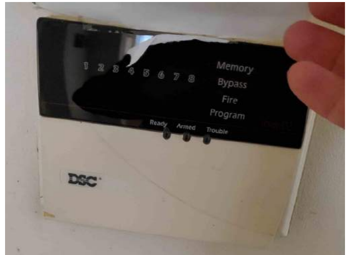
Figure 53 Security System Interface Panel
