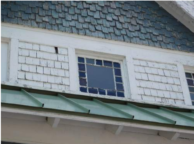
Figure 10 West gable showing typical wood shingle condition. The inner faces of two parapet walls extending above the roof line of the shed roof of the rear addition are faced with fiber board siding panels. They are severely deteriorated at the roof line and exhibit paint loss.
