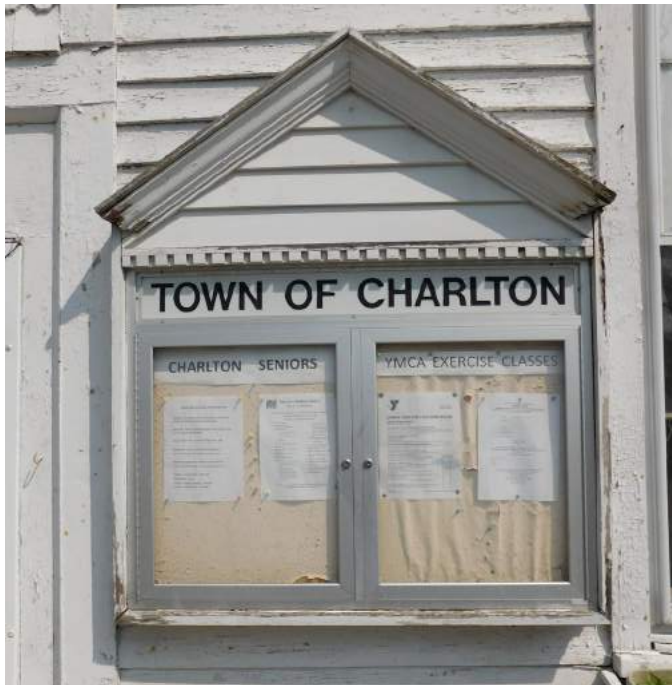
Figure 15 Rotted wood display board case.
