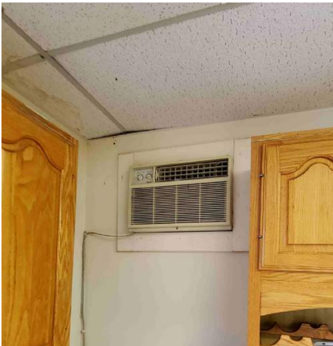
Figure 40 AC Unit in Kitchen
