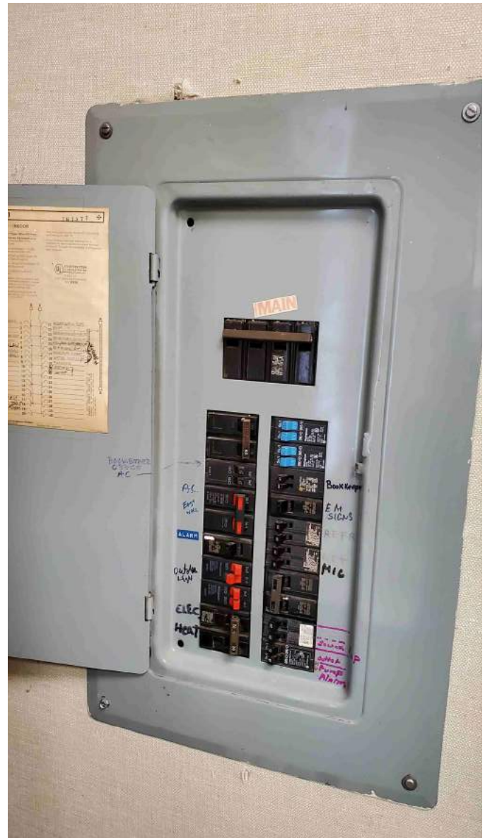
Figure 45 Main Electrical Panel
