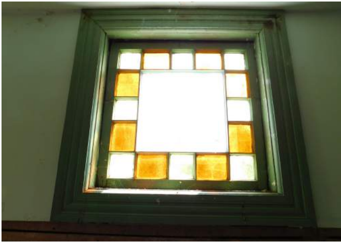
Figure 20 Typical square dormer window. This one exhibits two cracked panes and deterioration at the bottom left of the frame.
