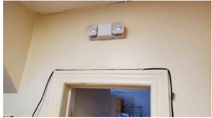
Figure 51 Typical Emergency Light
