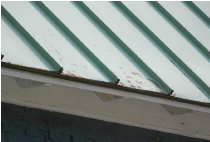
Figure 24 Typical minor corrosion at edge of metal roof.
