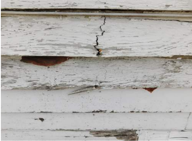
Figure 9 Typical paint loss and less common cracking and rot on weatherboards.
