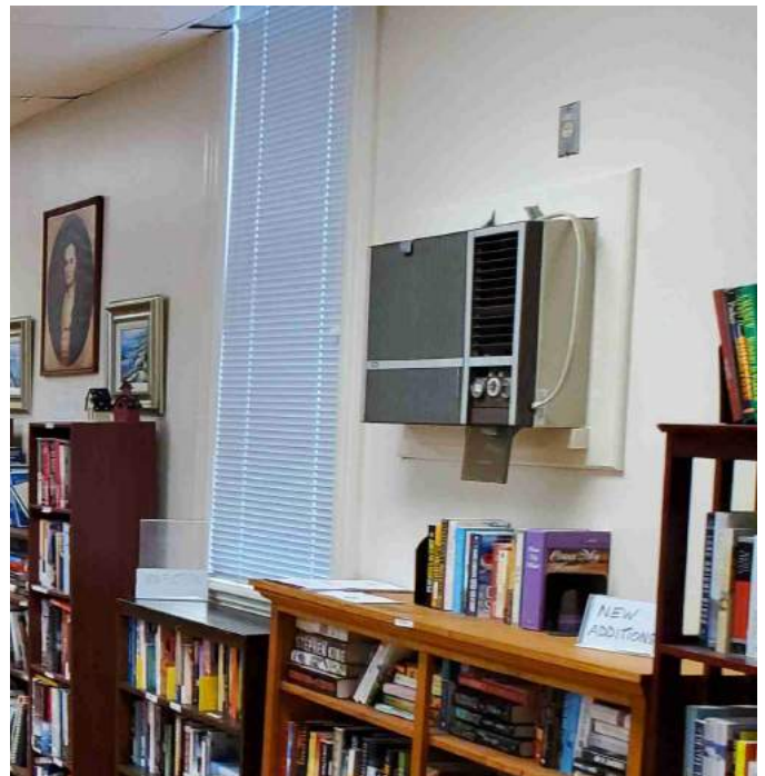
Figure 42 AC Unit in Main Room
