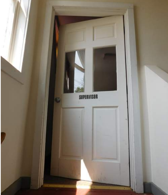
Figure 31 Second floor door with joint separation and marks.
