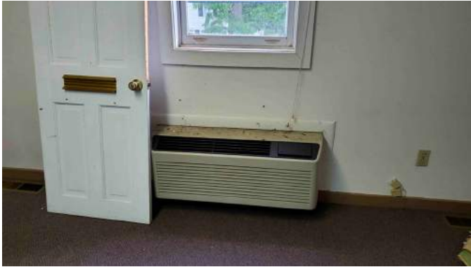
Figure 39 PTAC in Second-Floor Front Room
