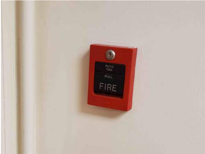
Figure 54 Typical Pull Station
