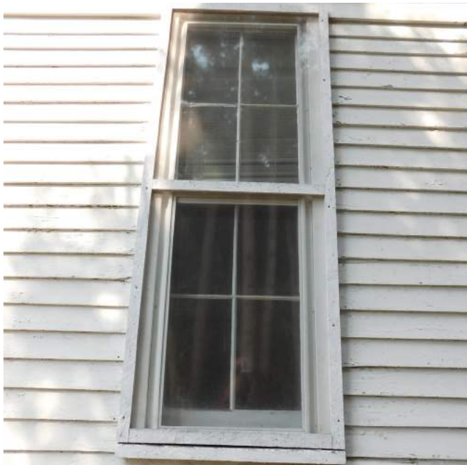
Figure 16 Typical four-over-four first-floor window. Note missing muntin in top sash.
