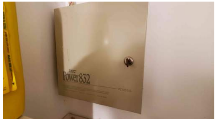
Figure 52 Security/Fire Alarm System Panel
