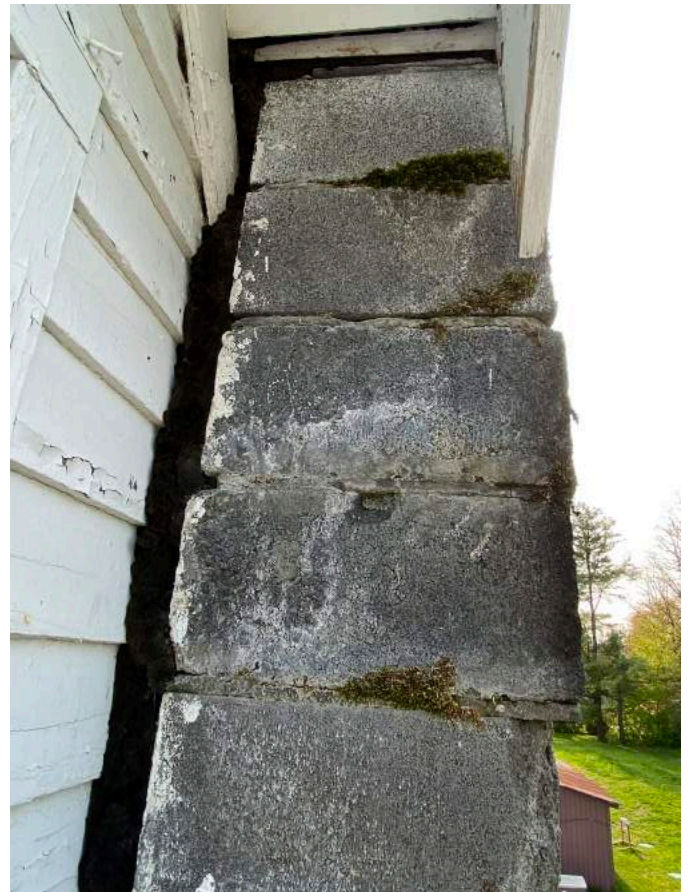
Figure 26 Detail of lower portion of chimney exhibiting a variety of material failures.
