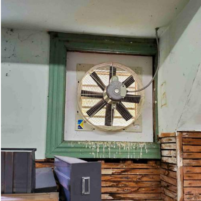
Figure 43 Second Floor Exhaust Fan
