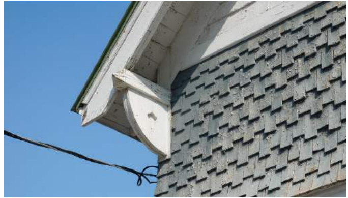
Figure 12 Typical bracket, fascia board, frieze board, and eaves showing paint loss.
