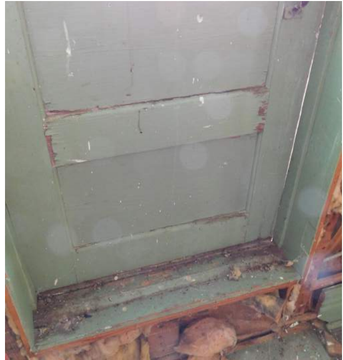
Figure 21 Bottom half of door leading to rear addition roof. Paint loss and rot at stile and rail meeting joints is due to water ingress from joint separation.
