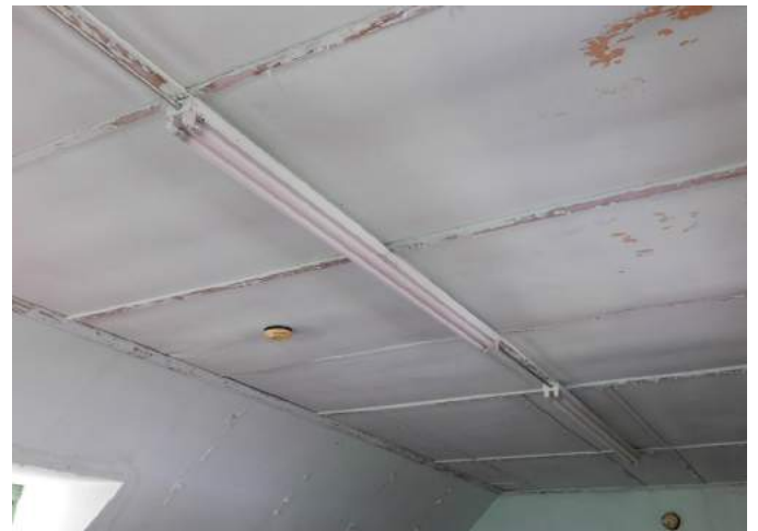
Figure 34 Warped gypsum board ceiling in second floor hall. Note paint peeling, particularly on battens.
