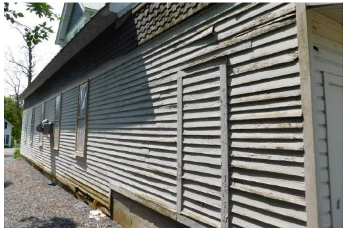
Figure 8 Deteriorating weatherboard on east elevation. Note also deteriorated former door casing.
